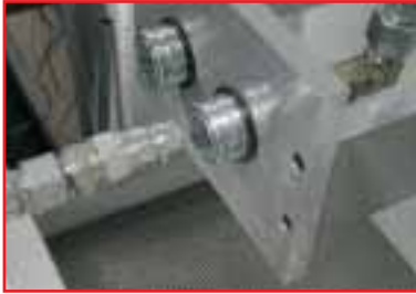
On the wall, with blocked sleeve and hose with coupling
